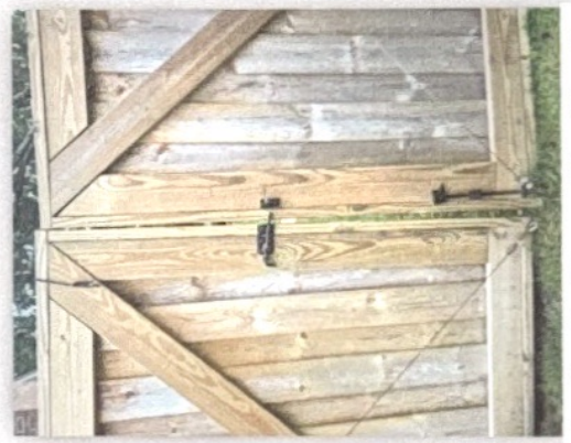
Looking South toward Front Street, Doors sagging at center.
