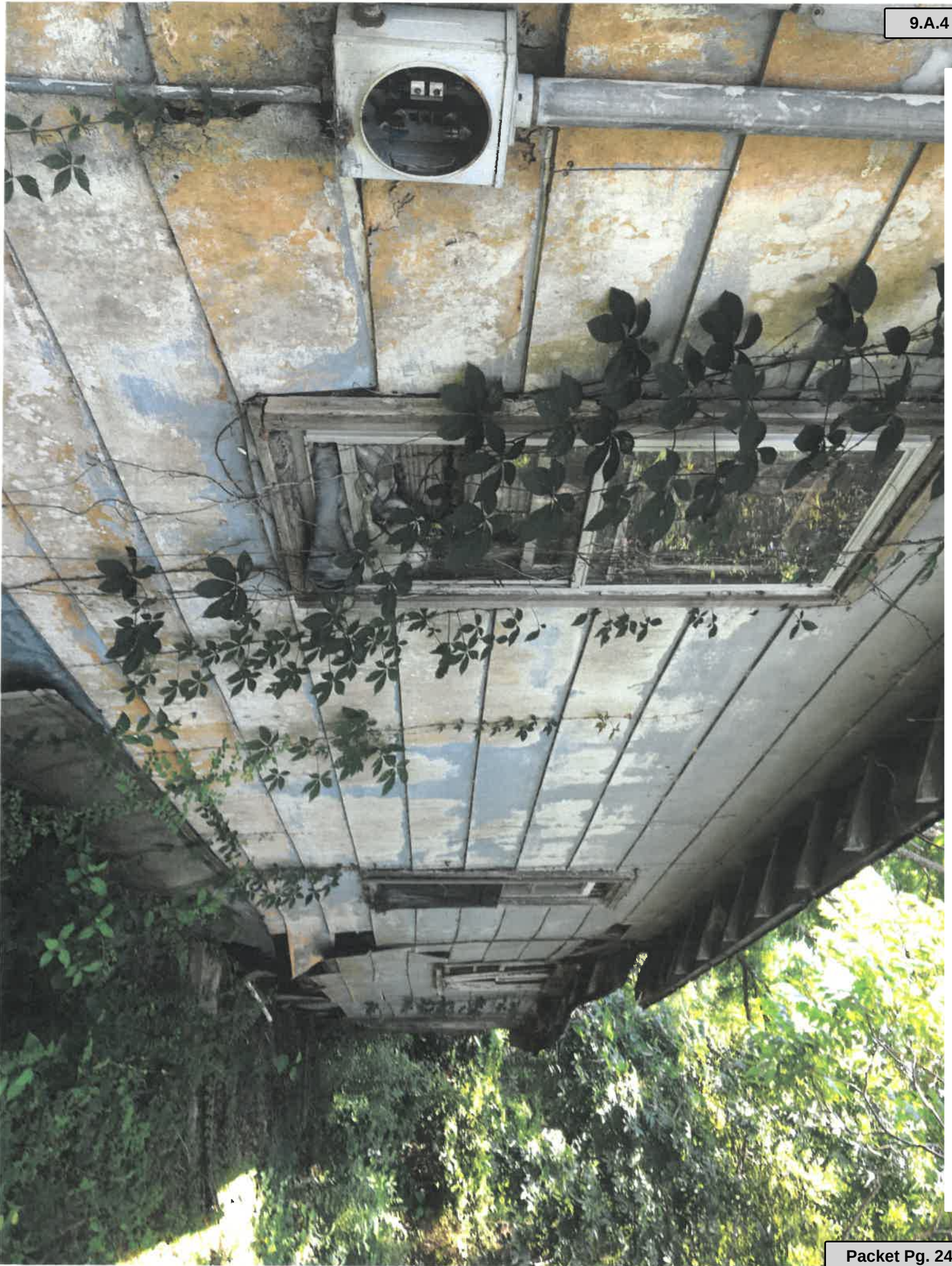
Attachment: 1925 Gilbert St (3094 : Complaint Petitions for Dilapidated Structures)
