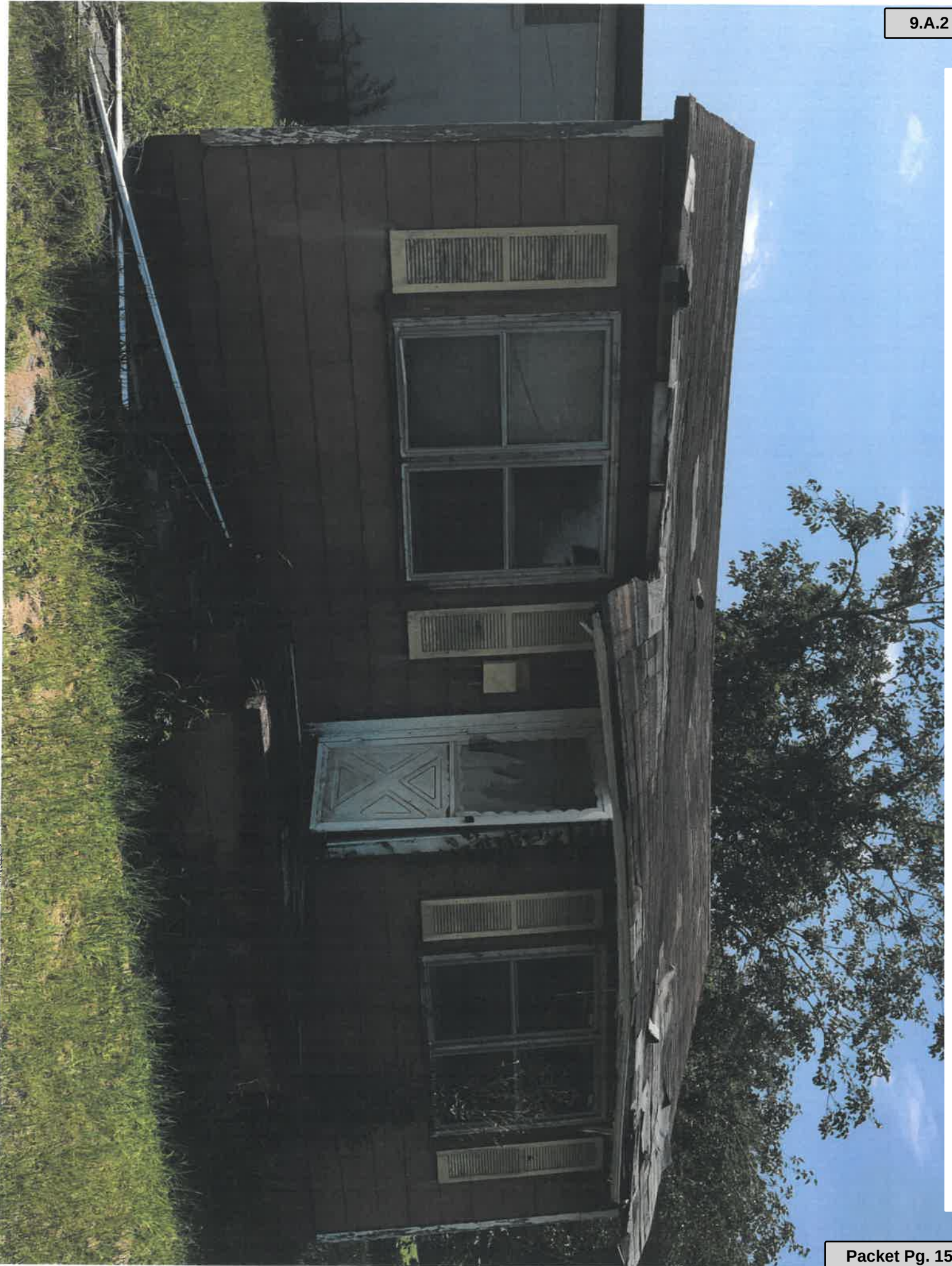
Attachment: 505 Duke St (3094 : Complaint Petitions for Dilapidated Structures)
