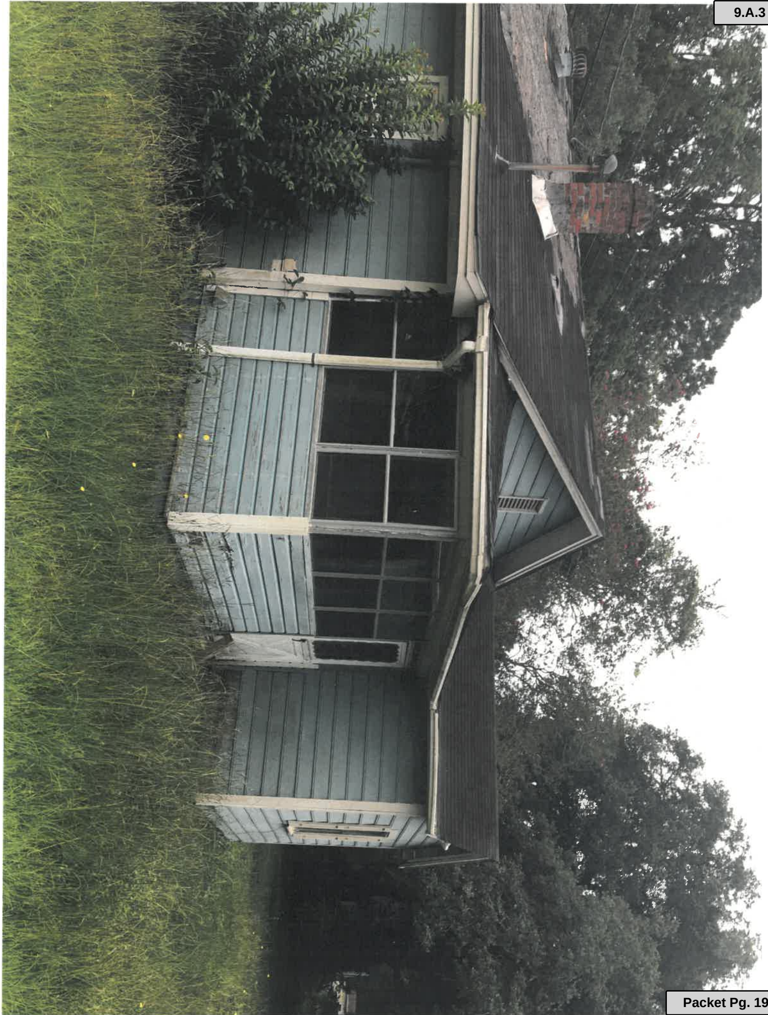
Attachment: 915 N Congdon St (3094 : Complaint Petitions for Dilapidated Structures)
