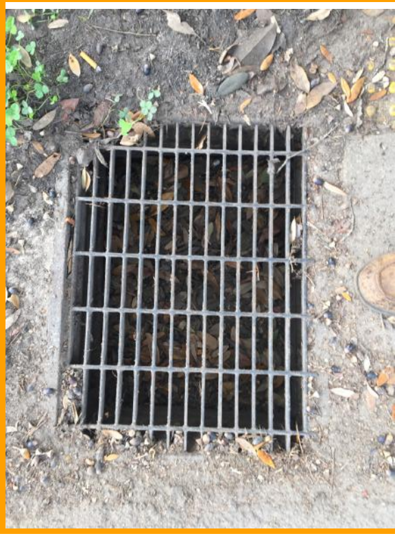
2 Existing drain at the intersection of North Congdon and Duke Street. Drain is clogged.
