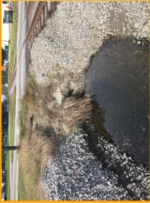
6 Existing collapsed drain pipe under North Congdon Street near the end of the project. Photograph taken facing NW.
