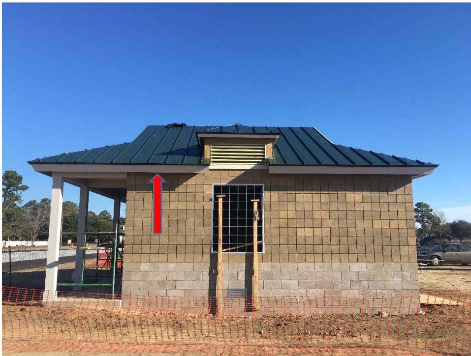
Photo No. 2 Description: Right Elevation. Arrow points to roof soffit which lacks perforated panel at the bottom.
