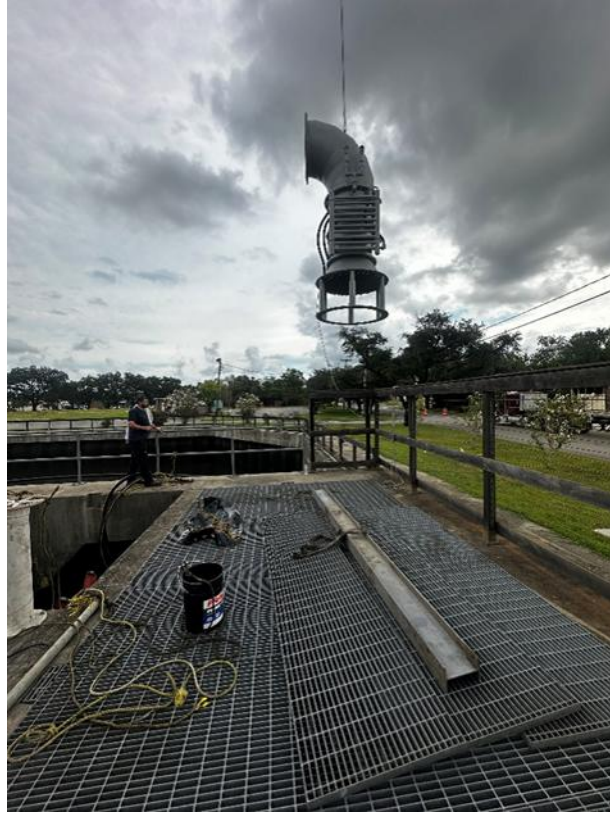
Figure 12 – Existing MWI hydraulically-driven submersible pump installation
