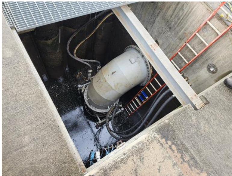
Figure 3 – View of existing MWI hydraulically-driven submersible pump in wet well
