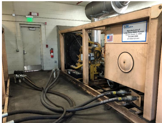
Figure 5 – Existing Diesel Engine Driven Hydraulic Pump in Motor House
