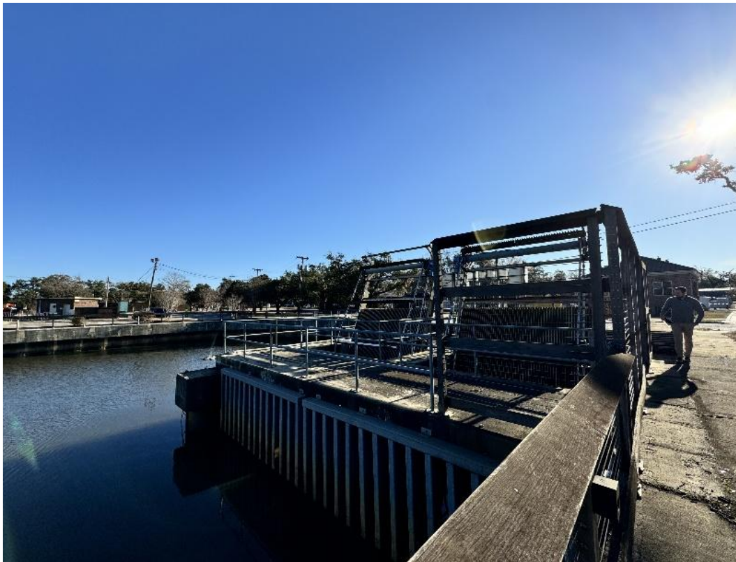
Figure 1 – Existing Bar Screens
